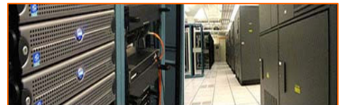
Picture courtesy of 365 Main
